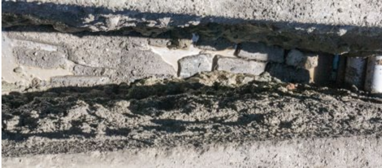
The historic brick street visible approximately 4 feet below Townsend St in the slot trench west of 4th St excavated on July 18, 2024
