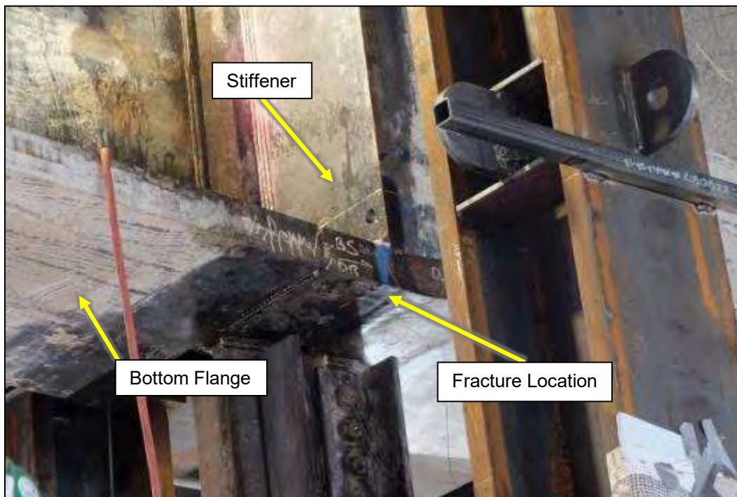
Fig. 3. Typical location of north side girder fracture, where the fracture was protected with silicone prior to flange sample removal.
