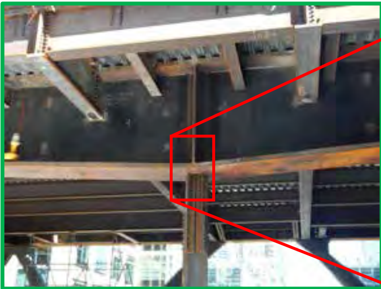
2. Hanger-to-girder connection at site of fracture (before fracture)
