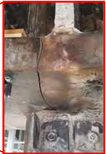
3. Fracture through bottom flange
