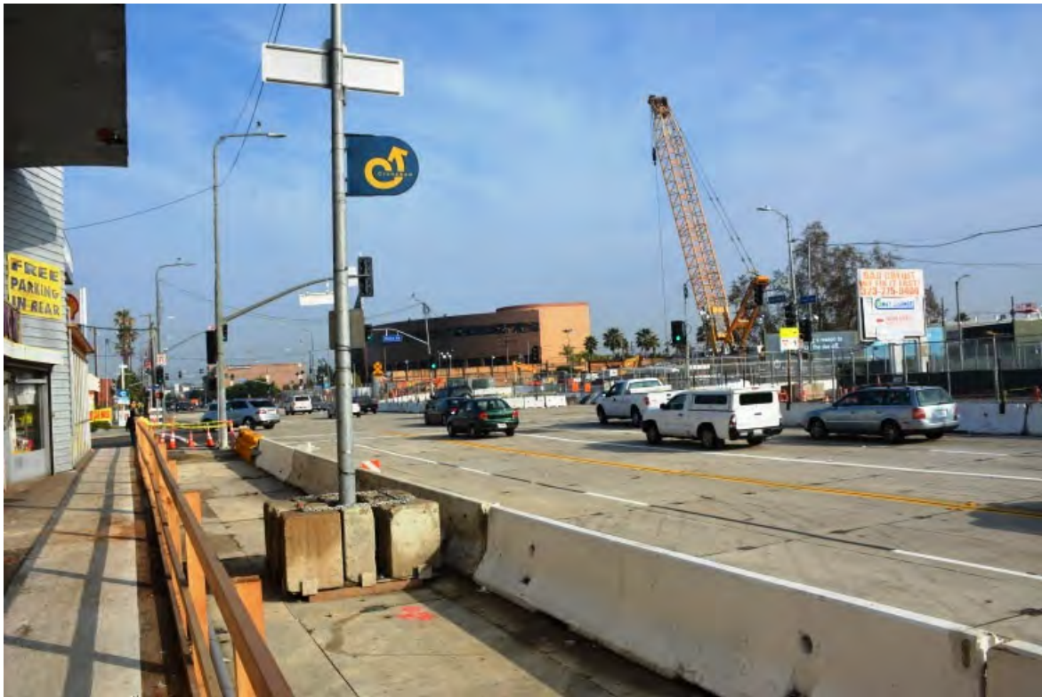
Figure MR-3. Photograph of Traffic Flow Over Decking While Excavation Continues Below
