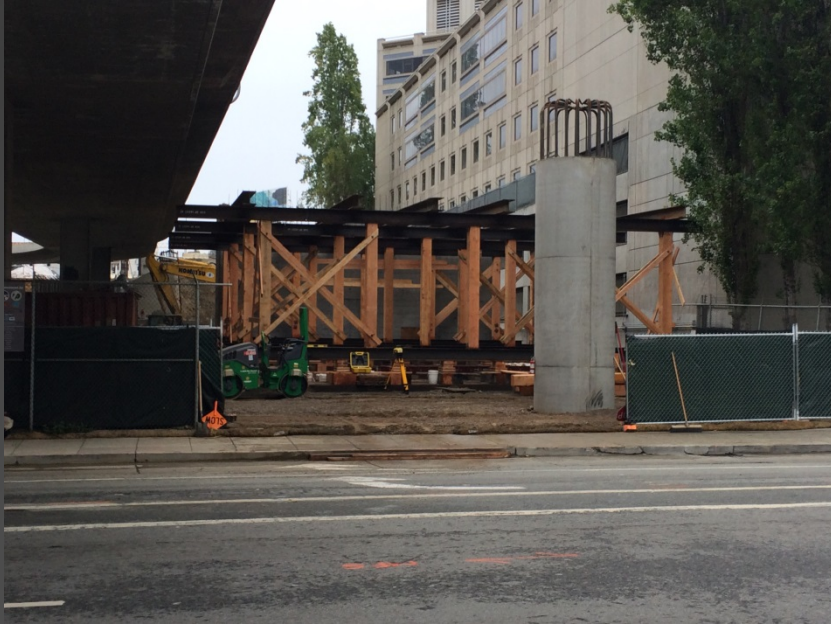
Above Left and Right : Falsework erection in progress, southside of Folsom Street.
