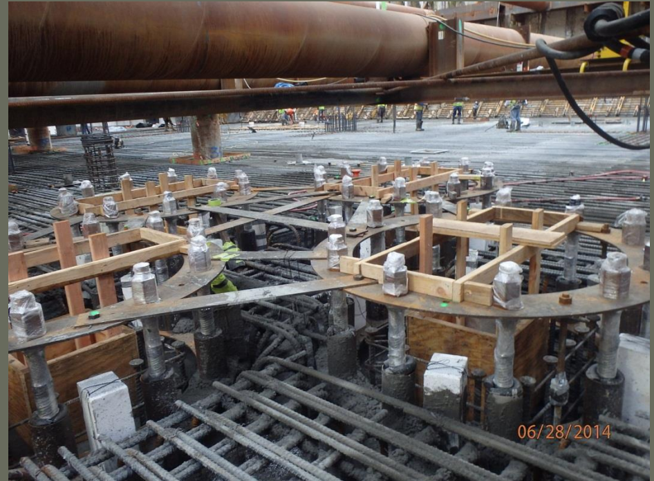
Light Column Anchor Bolts.
