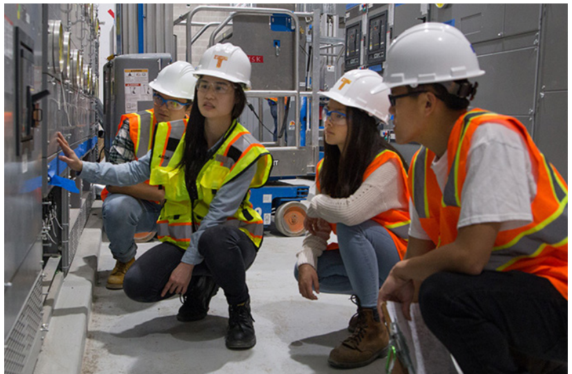
Interns Danielle Lei, Morgan Mosqueda and Nathan Zhou visit the main switchgear room with electrical engineer Patty Polpattana.
