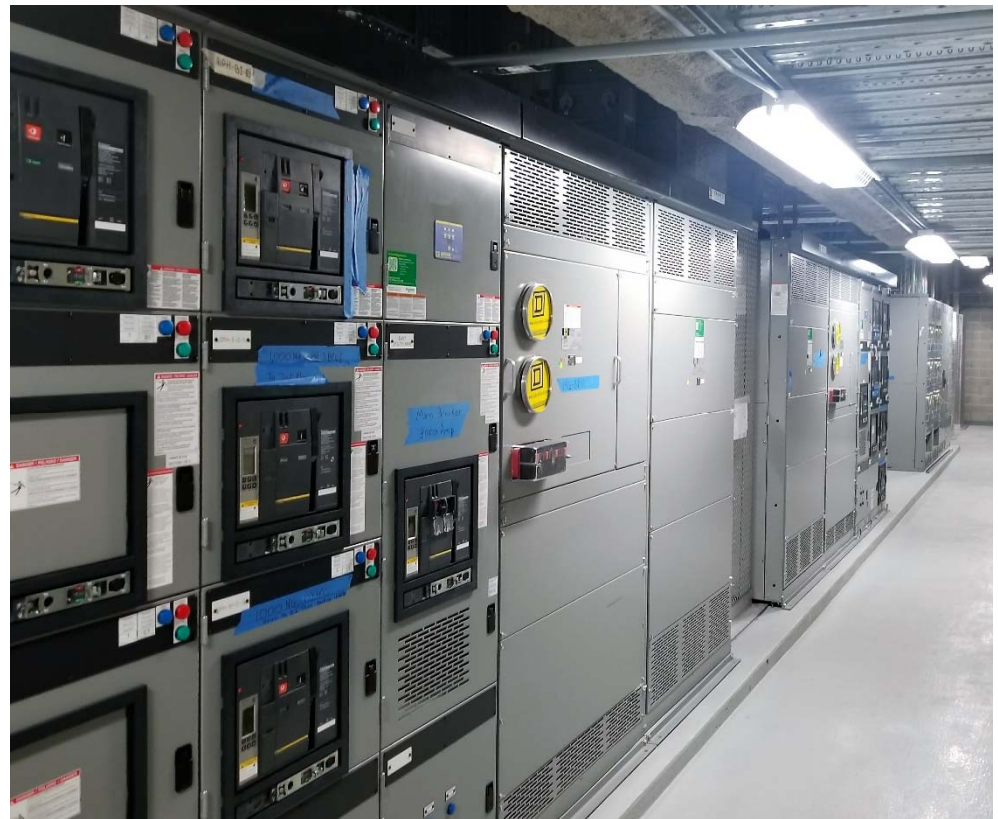
Switchgear Room B1561
